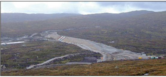
The new Glendoe pumped storage scheme. This shows the dam under construction to create a high altitude reservoir (over blanket peat).
