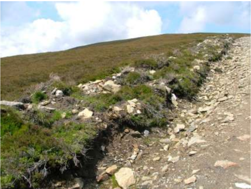
Below: Damaged verges on track near Ballater
