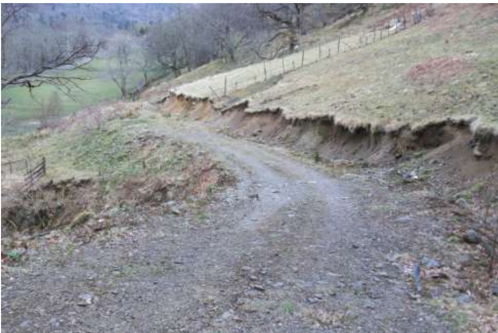
Below: Eroding verges near Loch Creran
