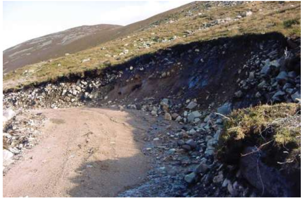
Above: Eroding bank, Cairngorms National Park
