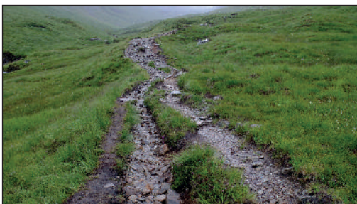
An eroding path above Bridge of Orchy.
