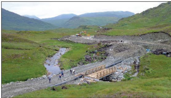
One of the new run-of-river hydro schemes in Glen Falloch under construction, within the Loch Lomond and The Trossachs National Park.
