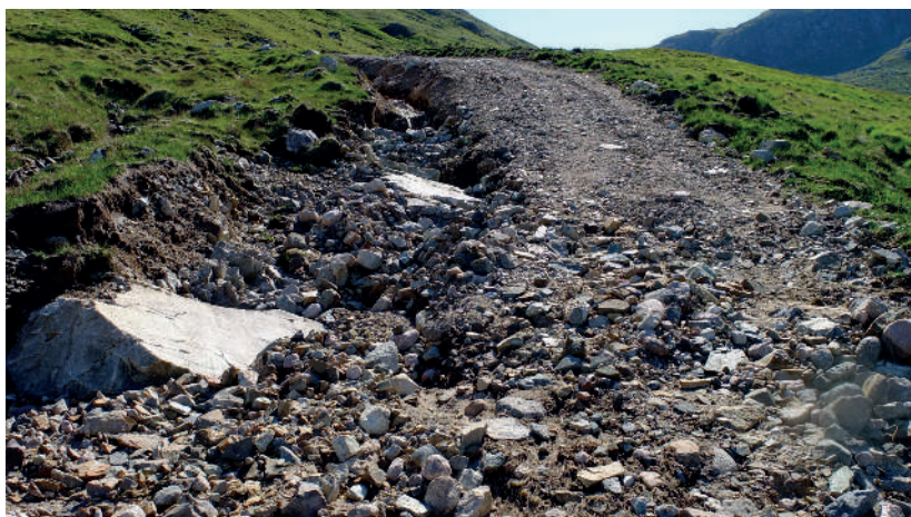
A badly constructed track below Ben Sgulaire, showing water erosion. Photo James Fenton
